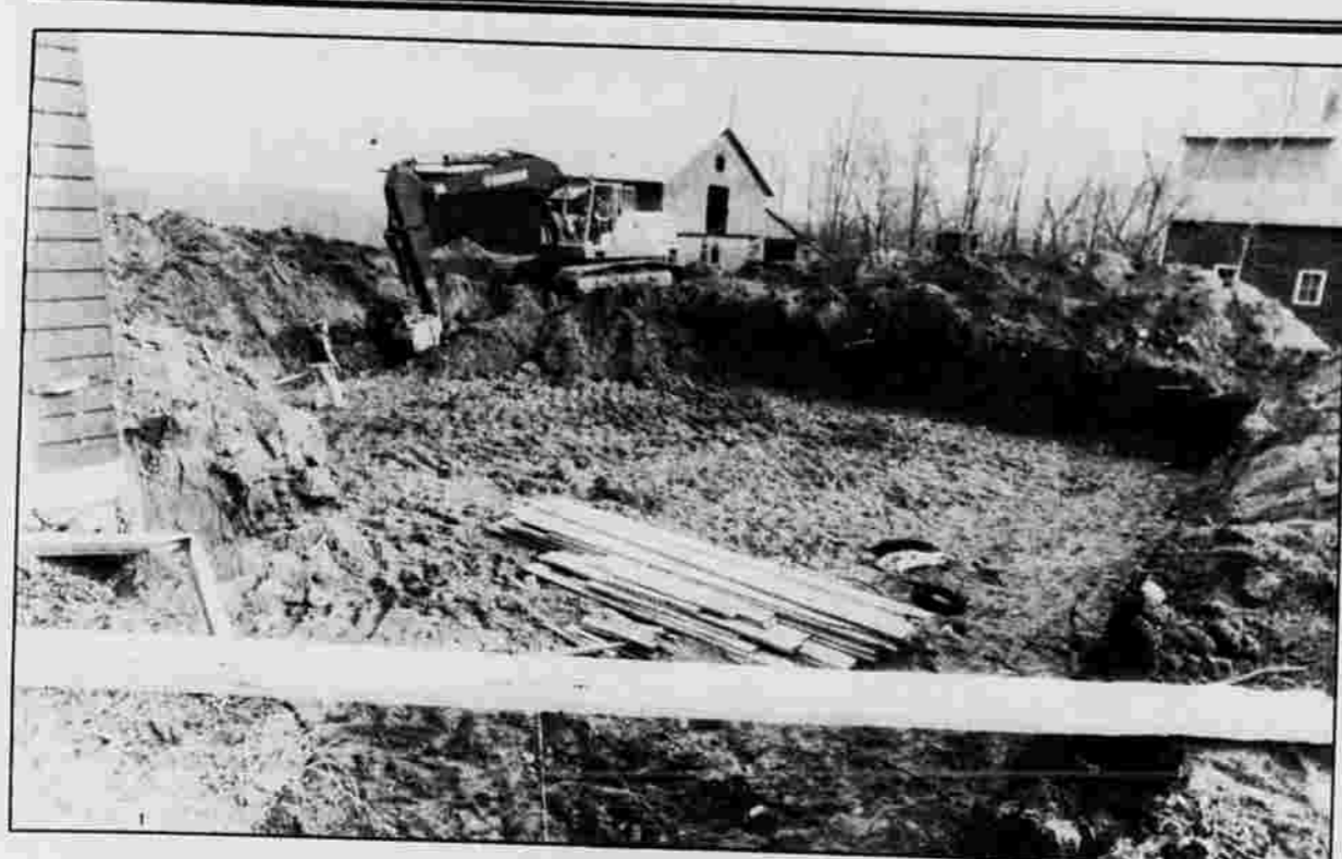
IT'S GONE — A colonial-style home will be built on this site on High Street in Coventry. An old farmhouse on the site was demolished Tuesday without a permit.
